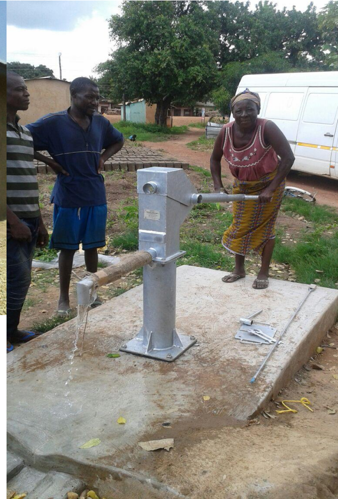
A newly constructed borehole at Fian processing centre for provision of portable water for butter processing and community use
